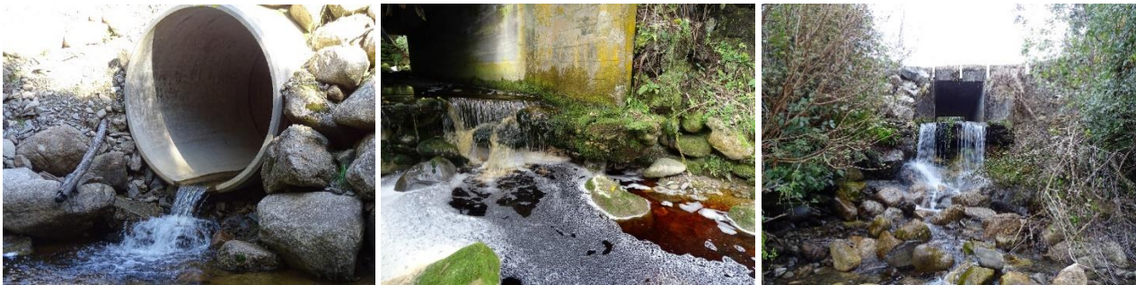
Figure 5: Culverts Impeding Fish Passage
