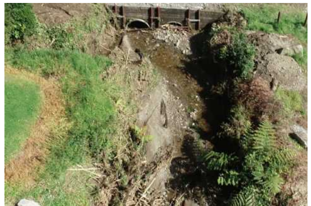
Figure 16. Blocked culverts may have been partly responsible for some of the observed debris inundation in Granity. Photo: BDC.
