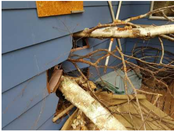
Figure 10. Trees pushed through an external wall of a house impacted by landslide debris (example from Marlborough)
